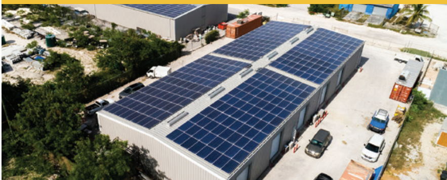
One of several grid-tied solar PV systems that FortisTCl has installed on commercial premises in Providenciales.
