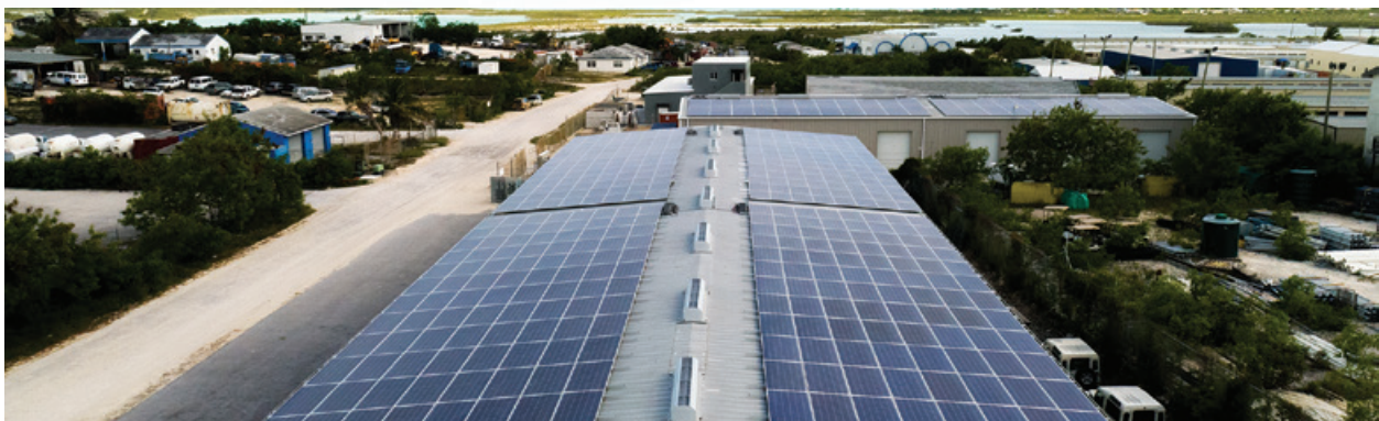
Approximately 0.5 MW of solar PV systems are currently installed on the FortisTCl grid, representing a range of commercial customers.
