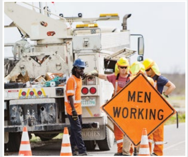
>> FortisTCl Junior Plant Operator Corean Kelly and visiting utility workers from Newfoundland Power discuss their next move during restoration on South Caicos.
