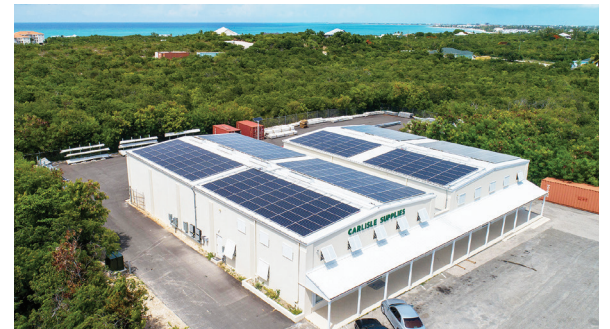
A large commercial installation at Carlisle Supplies on Providenciales, one of nine participants in the FortisTCI Utility Owned Renewable Energy (UORE) Program.
