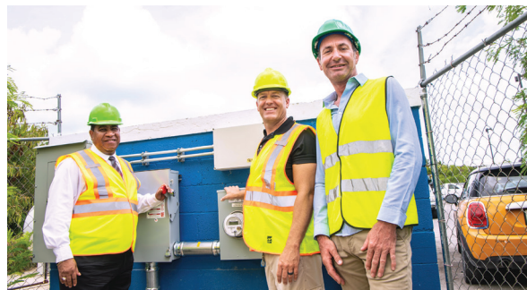
FortisTCI President & CEO Eddinton Powell shares a moment with owner of Grace Bay Car Rental Todd Foss (center), and Green Revolution's Robin Spruce following installation of Grace Bay Car Rental's solar PV to the grid.
