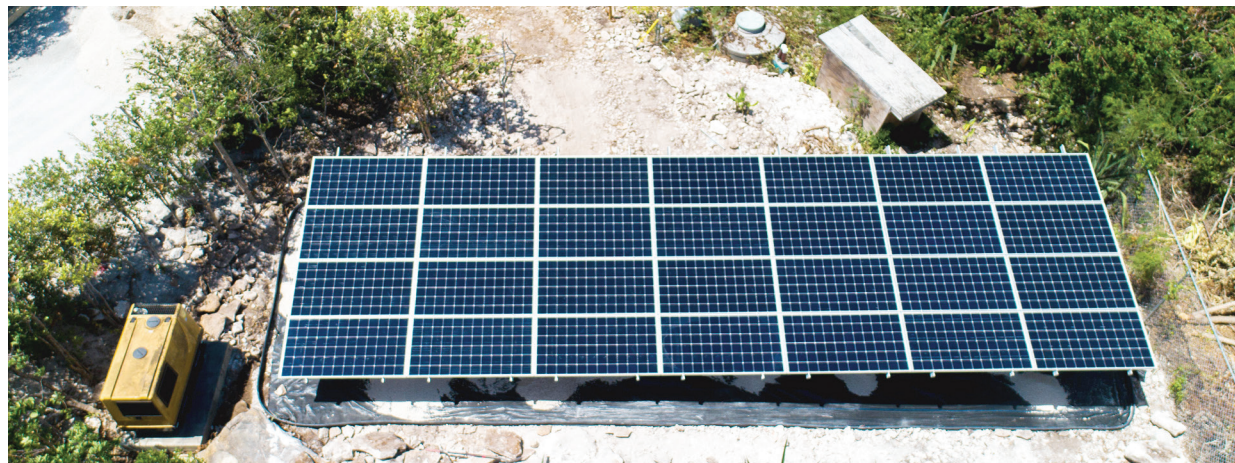
This solar plus battery installation at a residential property in Providenciales is part of a pilot project that FortisTCI is undertaking to determine the suitability of the technology for the company's renewable energy programs.
