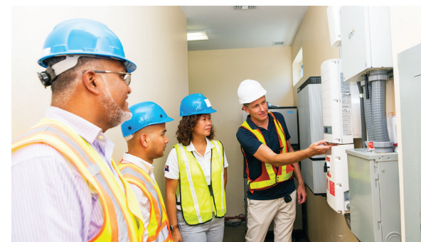
Battery storage technology, installed at FortisTCI's Providenciales plant, is part of a pilot project that was launched in August 2019. The project will gather data to guide the company's renewable energy programs relating to energy storage.
