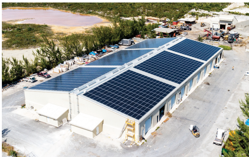
At 397 kW, FortisTCI's solar PV project at Caicos Depot, Providenciales, is the largest single installation under the company's Utility Owned Renewable Energy program.
